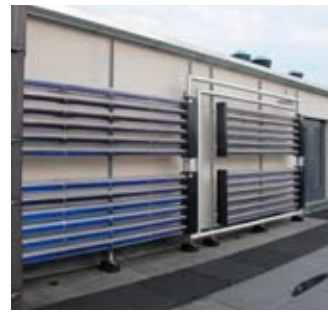
Renewable energy: solar thermal at the BREEAM Excellent Standard Lennard Jones laboratory.
